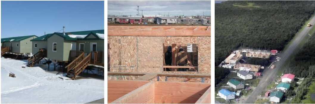
AVCP Projects From left: Chefornak teacher housing, new construction in Chevak, AVCP projects in Alakanuk
